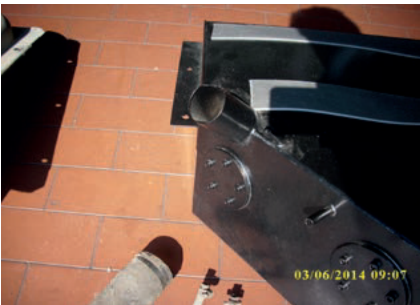
Tank neu - Anschlüsse
